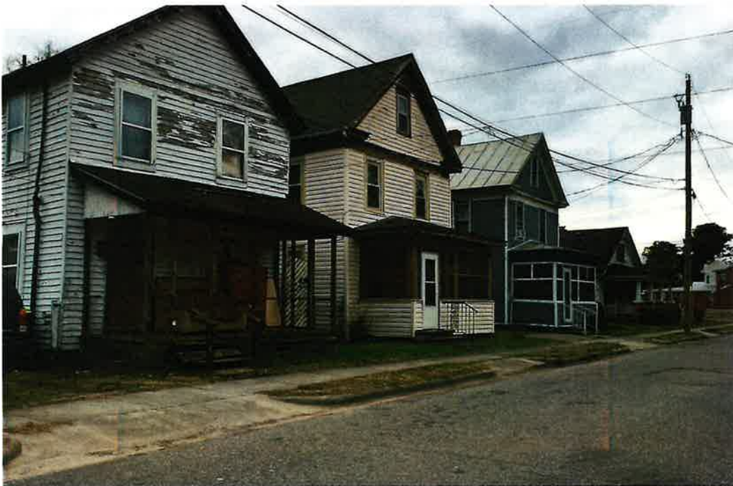
A section of Dobbs Street showing the predominant house form in Uptown Hertford
